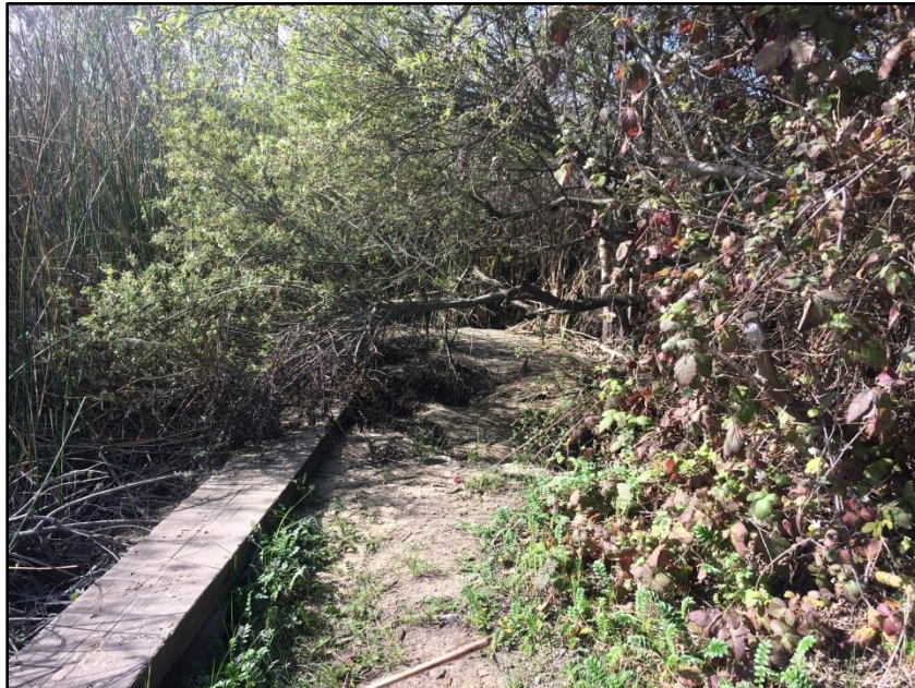
Photo 2. View south of existing pipeline alignment within the Oceano Lagoon and existing pedestrian trail (April 10, 2018).
