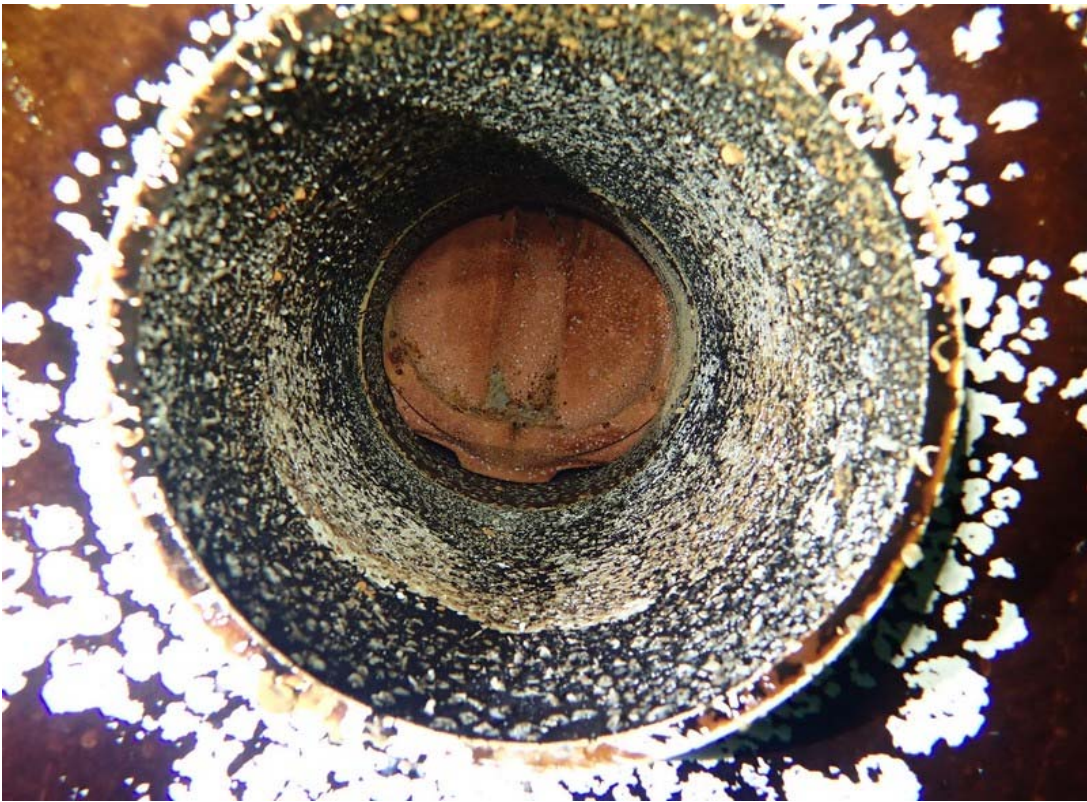
Interior view of the shell nozzle on the right side of the top photo of this page. Blisters in the coating are visible as rounded white spots. Minor corrosion is present.
