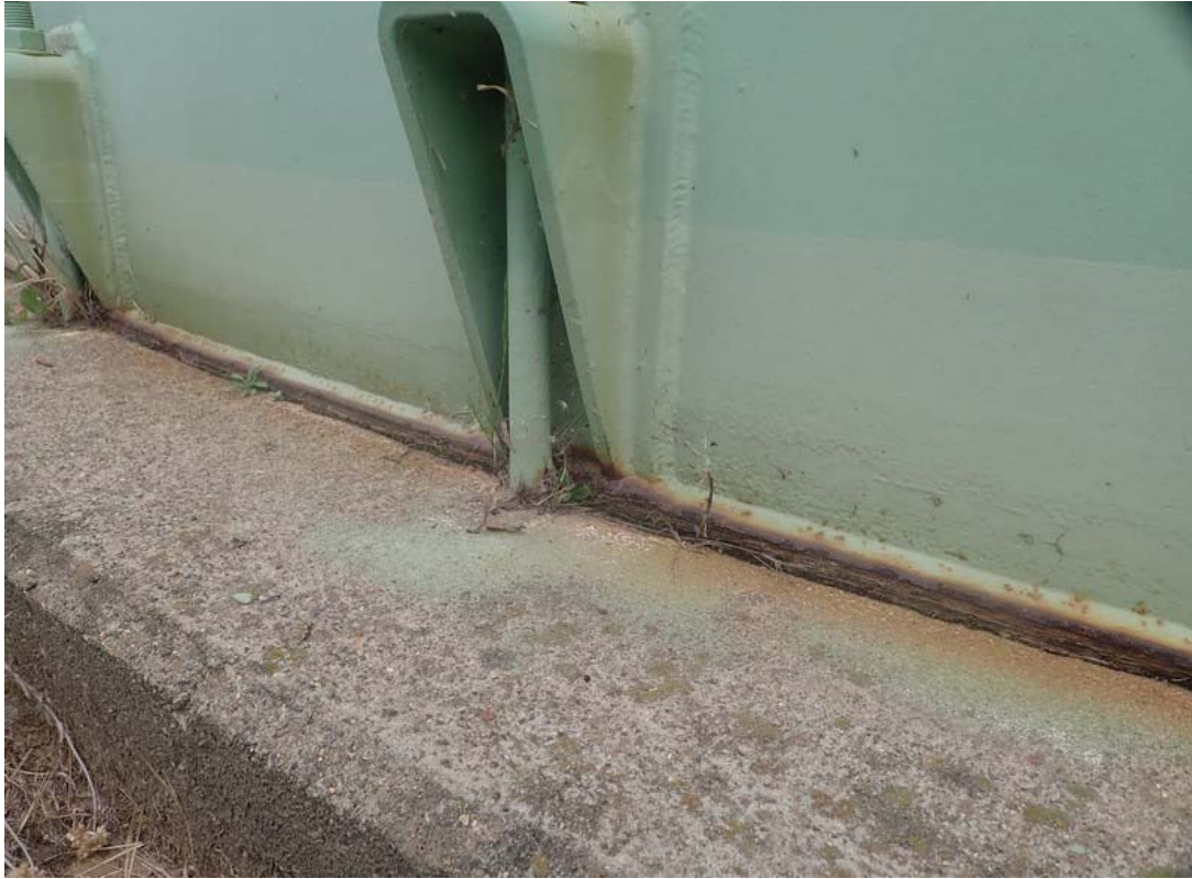
This view shows a typical mechanical anchor along with lower shell. Significant corrosion is present.
