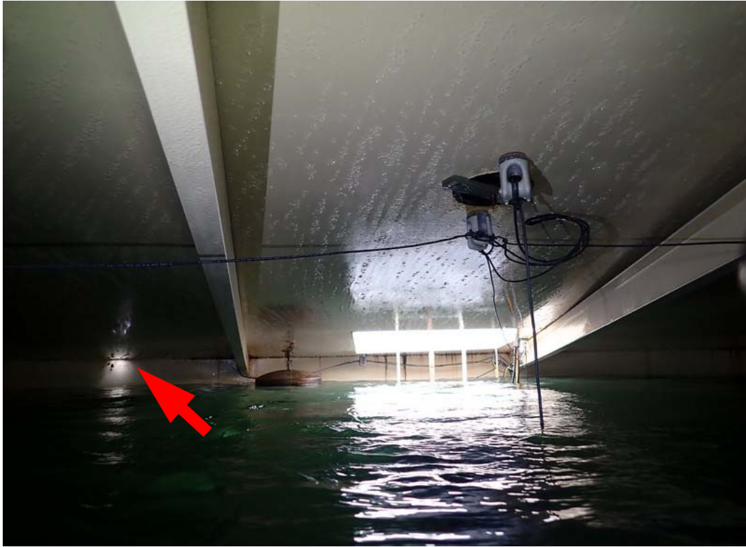
View of the roof hatch from the interior. The arrow indicates the location of a hole that was sealed by ATS.
