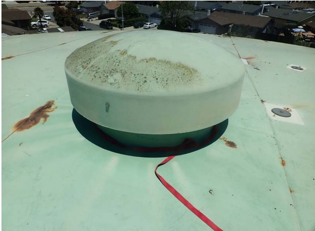
The roof vent consists of a fiberglass cover over a steel riser pipe.
