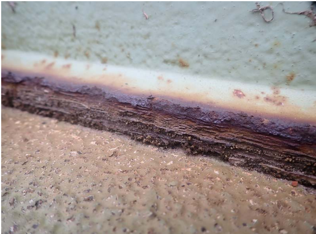
This close view of the exterior lower shell and bottom chime shows serious corrosion found on the outer edge of the chime. Continued corrosion here will eventually create a condition where bottom replacement is necessary.
