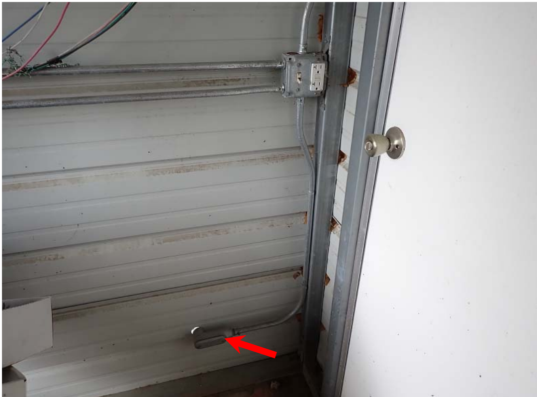
Apparent first junction box from the CP panel located in the well shed near the breaker box.
