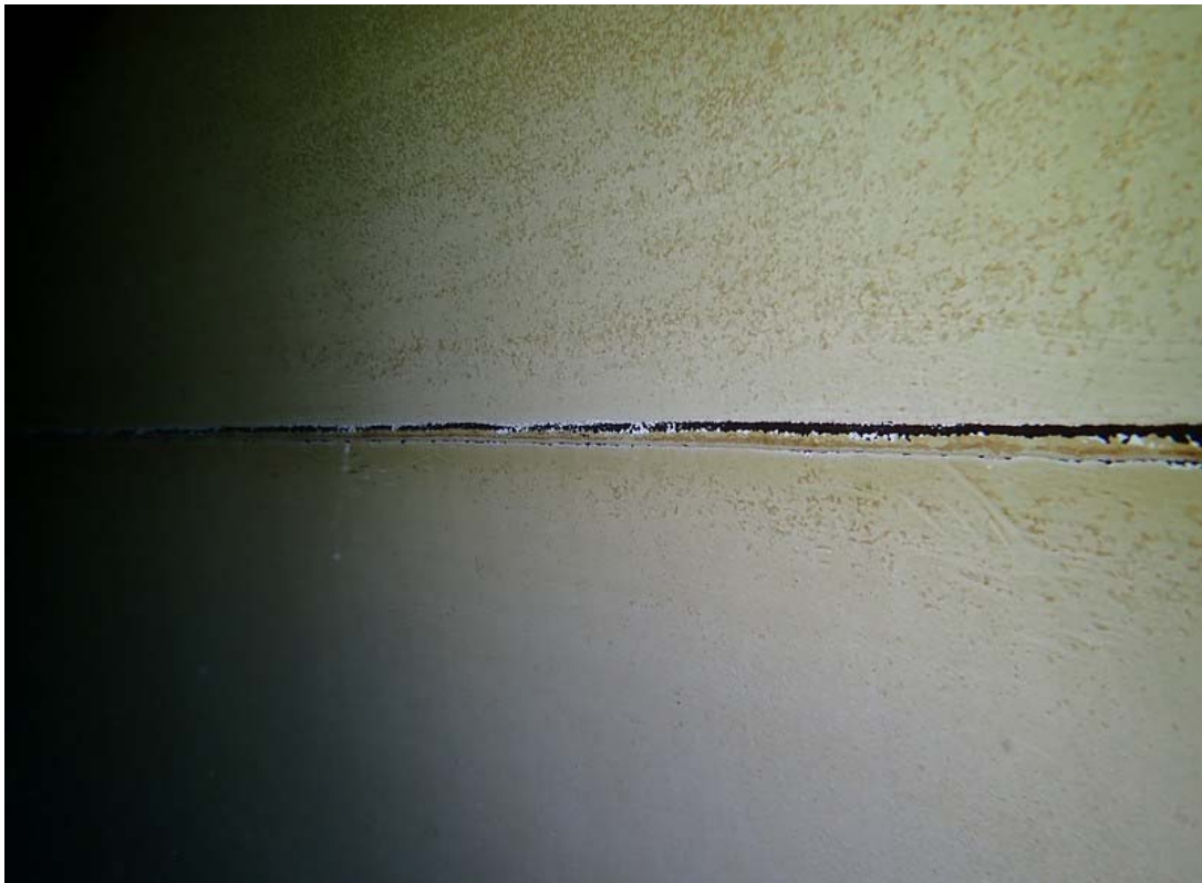
Interior shell in the submersion zone. This view shows a horizontal weld with sediment or staining visible along the top. The interior shell steel appears to be in good condition.
