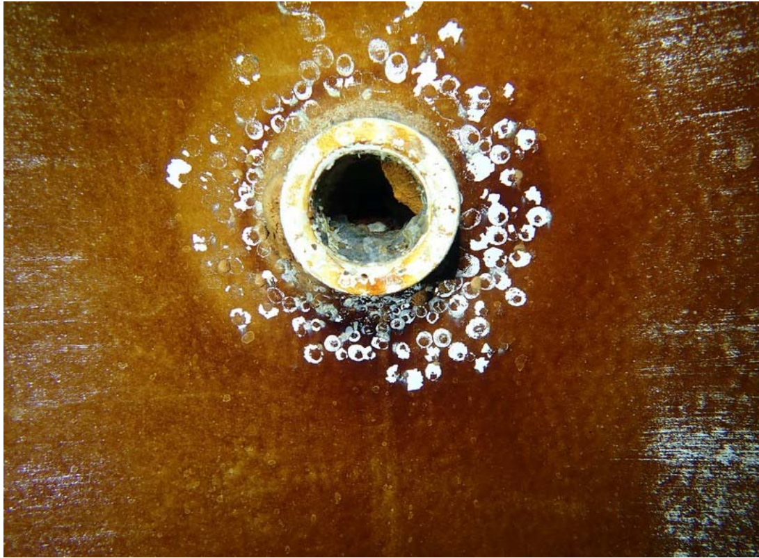
This view shows the interior side of the sample tap. Blisters in the coating are visible.
