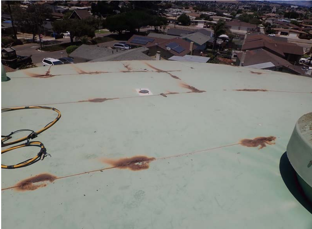
The exterior roof is the area with the worst corrosion on the tank. Approximately 50 locations have serious metal loss. ATS repaired the 10 worst locations that had holes where the 3/16inch thick roof has rusted through.
