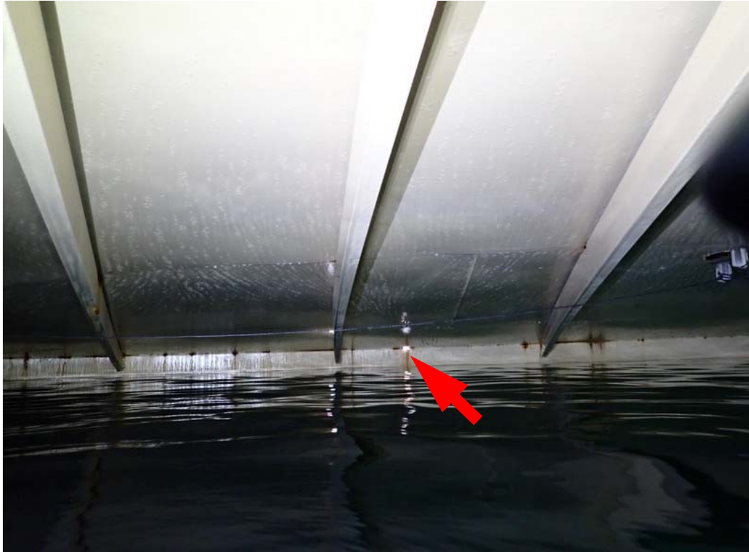
Interior roof plate and rafters. Broad view. Some minor bowing is present in the rafters. This view shows an example of nearly rust free plate but a hole is visible at the shell to roof joint (arrow). The hole was sealed by ATS.
