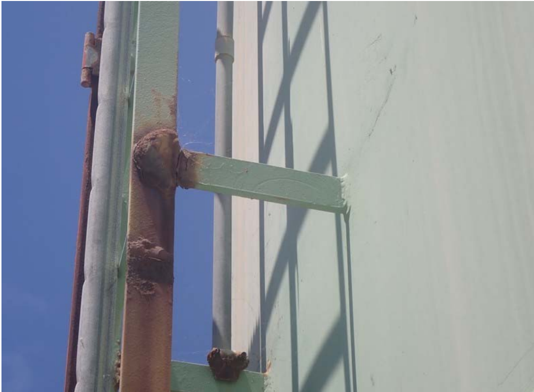
This photo shows one of several areas of serious corrosion on the exterior ladder.
