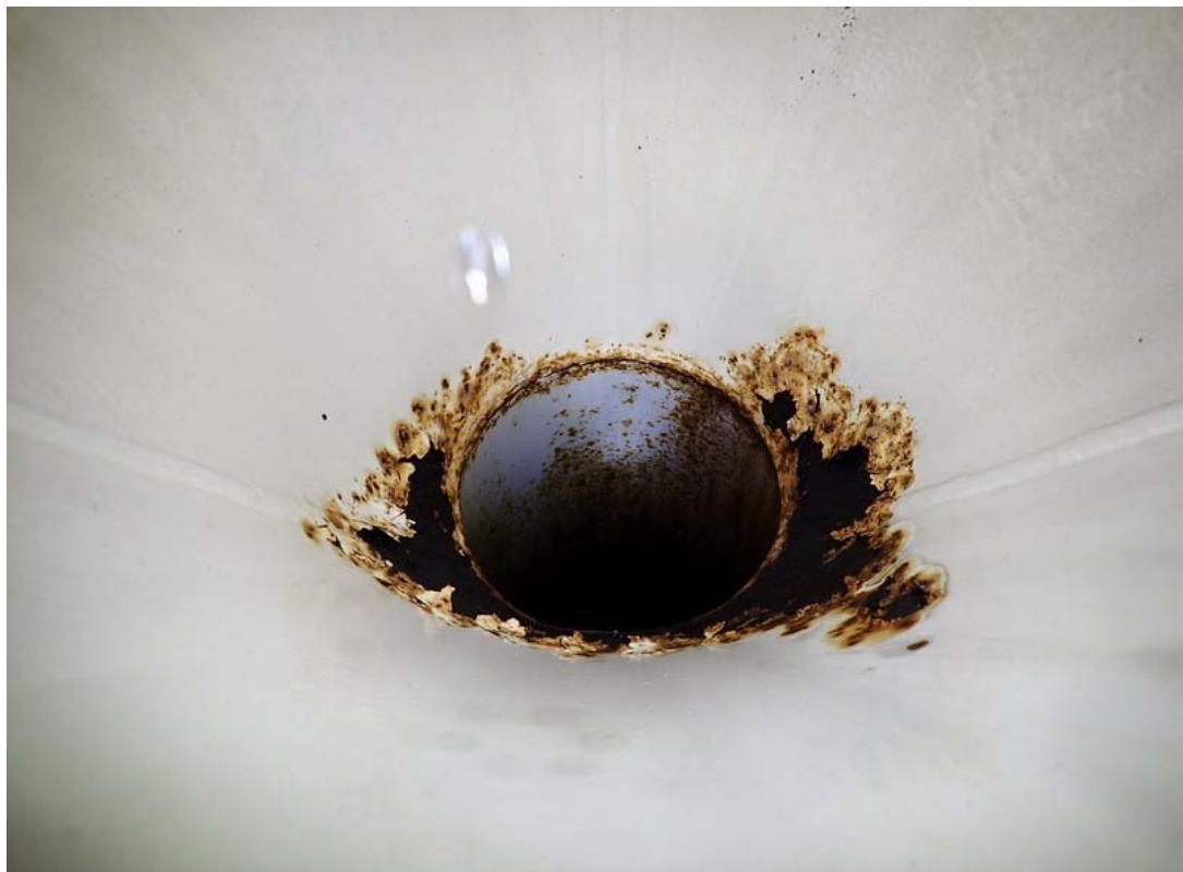
This view is of the inside of the overflow weir. Some corrosion is visible but the pipe appears to be free of obstructions.
