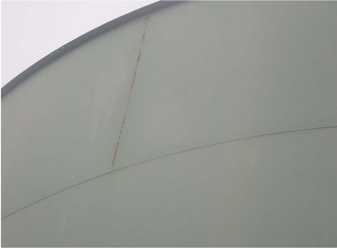
The upper shell and roof joint are shown in this photo. The coatings are in fair condition with significant aging of the coating and scattered corrosion.
